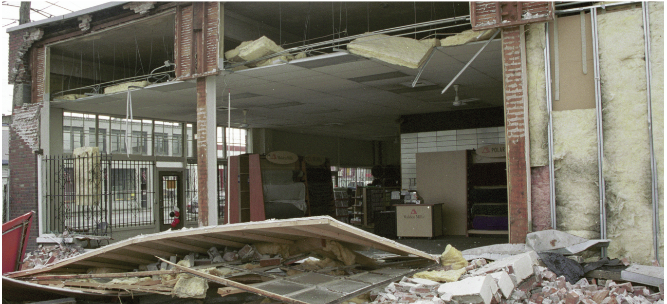
The Nisqually earthquake that struck Seattle, Washington, in February 2001 caused substantial building damage.
